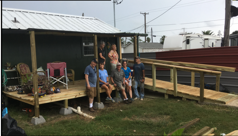
Handicap accessible ramp and deck built for Donna and her dog Mahi. This project was a challenge of mind, strength and endurance but Don Hartman had the right tool at every turn.
